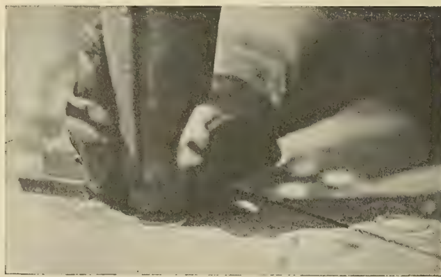
Fig. 16.—Driving Straight Down With Proposed Standard Set to Swell Rivet Shank and Fill Hole
